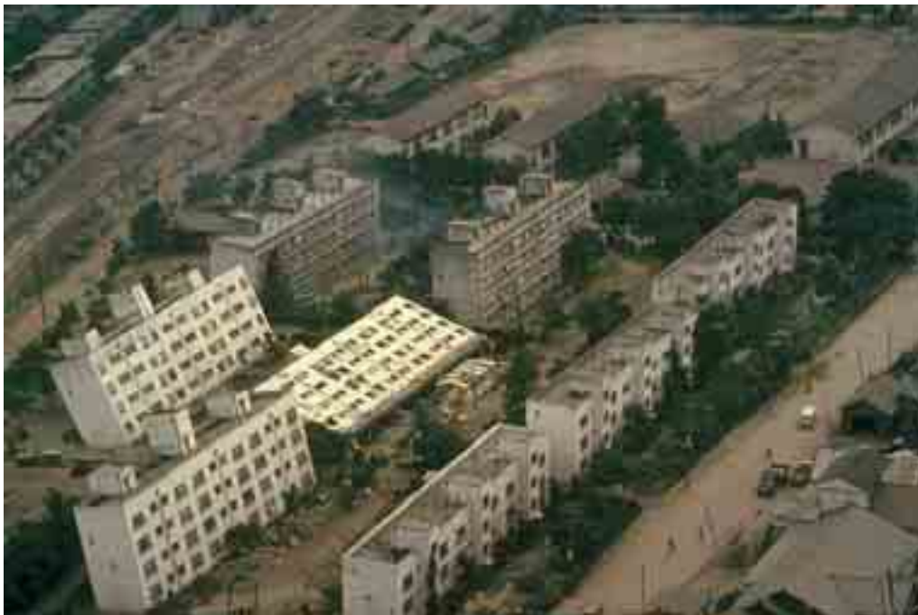
Figure A3.28 – Tilt of buildings at Kawagishi-Cho due to liquefaction following the June 16, 1964 Niigata (Japan) earthquake ( M_s 7.5). The preliminary estimate of the Inqua EEE Intensity is XI. Source: http://cee.uiuc.edu/sstl/education/liquefaction/
