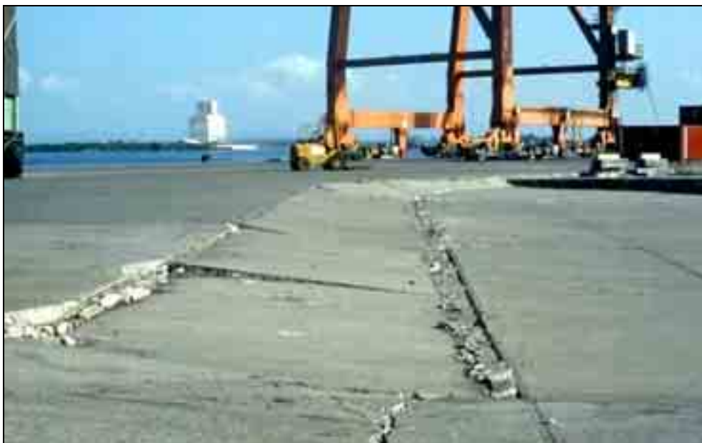
Figure A3.30 – September 19, 1985 Michoacan (Mexico) earthquake (M, 8.0): backfill compaction in the harbour facilities of Lazaro Cardenas. The preliminary estimate of the Inqua EEE Intensity is VIII. Photo E. Vittori.
