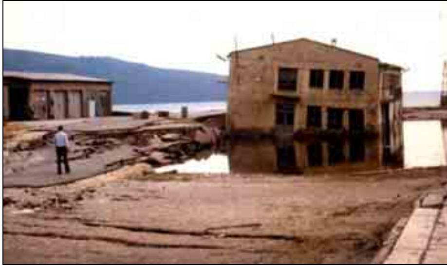
Figure A3.27 – Ground failure (liquefaction of artificial embankment) along the seacoast during the 15 April 1979 Montenegro earthquake ( M_w 6.9). The preliminary estimate of the Inqua EEE Intensity is X. Photo E. Iaccarino.
