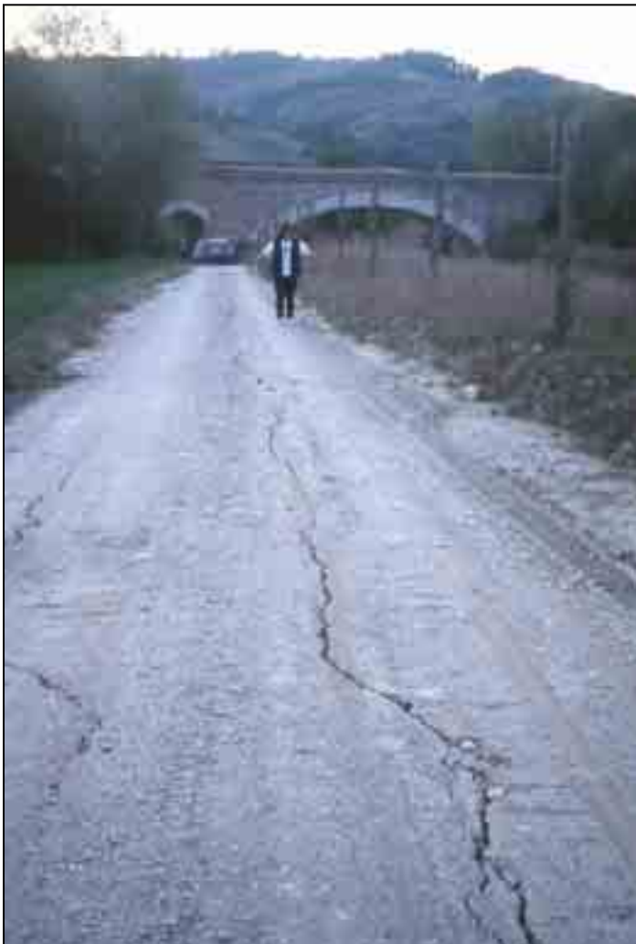
Figure A3.22 – Ground cracks affecting a dirt road in a flat area near Isola (Umbria region), caused by the 1997 Umbria-Marche (Central Apennines) earthquake (M w 6.0) (Esposito et alii, 2000; Vittori et alii, 2000). Photo S. Porfido.
