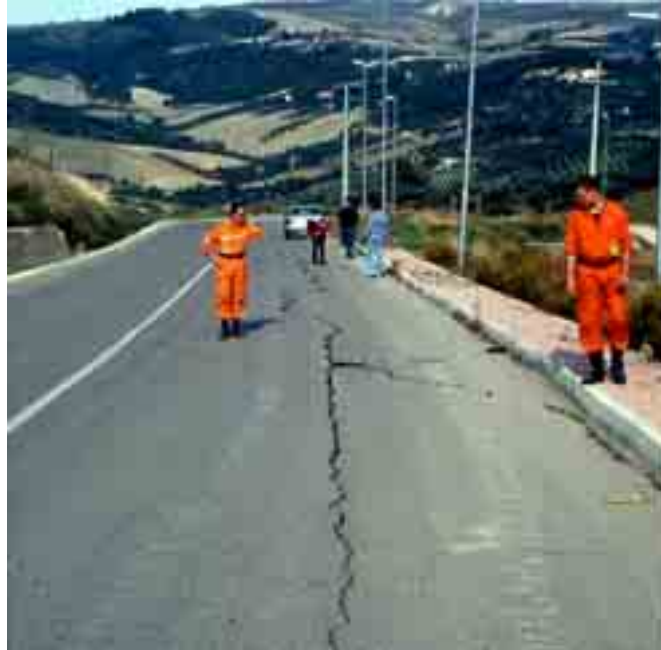
Figure A3.23 – Ground cracks of debated origin affecting a paved road near San Giuliano (Molise region), caused by the 2002 Molise (Southern Apennines) earthquake (MI 5.4). Photo E. Esposito.
