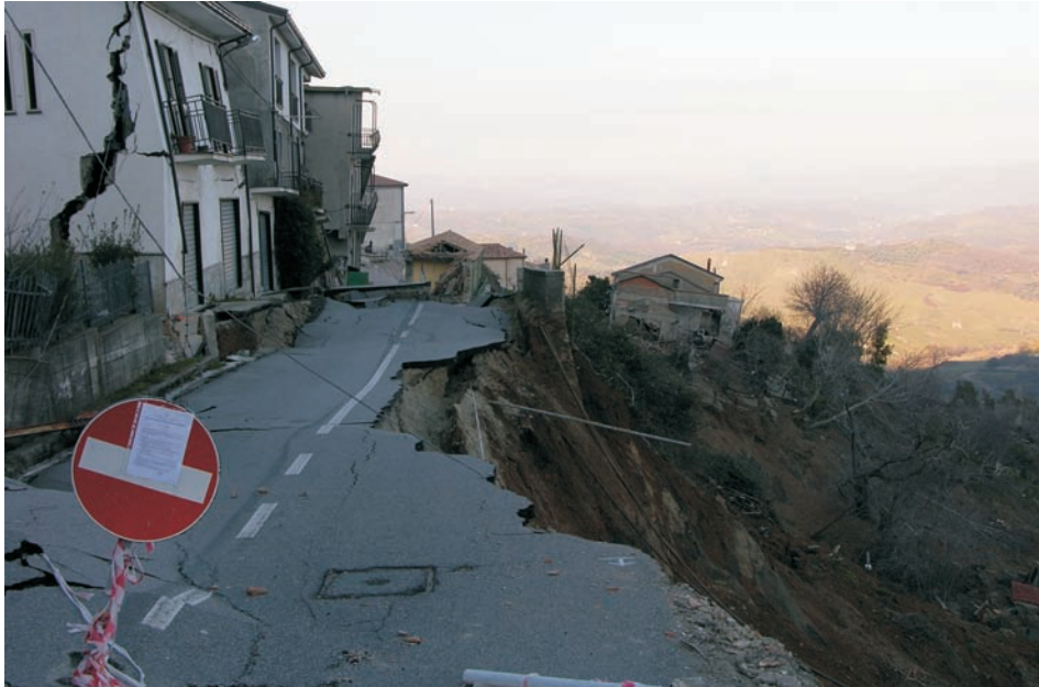
Figure 16: Damage to the village of Cavallerizzo, Cerseto Municipality (Calabria Region), March 7, 2005
