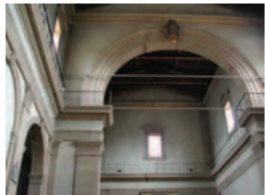
Figure 6 - The interior of San Salvatore al Monte: on the arch, some old restored cracks are evident.
