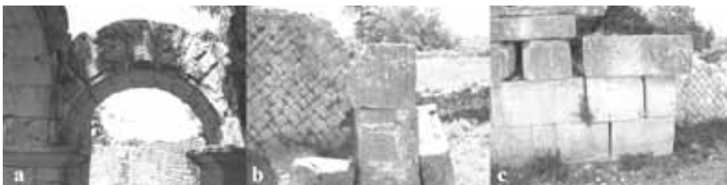
Figure 8 - Three examples of disconnected structures due to earthquakes: a) off-setting of lithons in an arc; b) block rotation in a pillar; c) increase of spacing between blocks in a wall.
