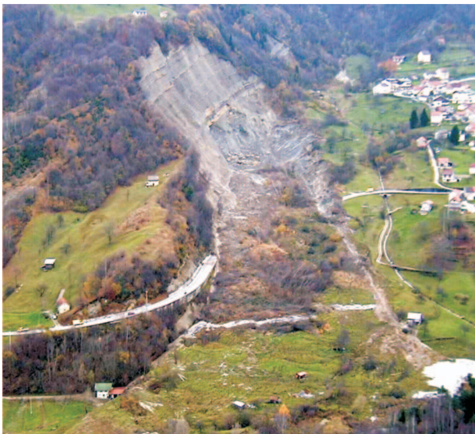
Figure 17: Landslide at Borsoi, Tambre Municipality (Veneto Region), reactivation in autumn 2000 and in May - June 2004
