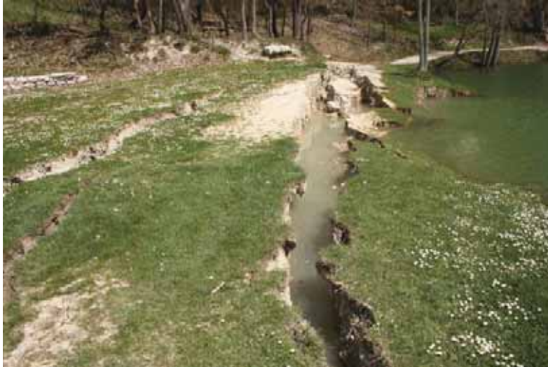
Fig. 7 - Sets of cracks dislocating the shore on the northern margin of the lake.
