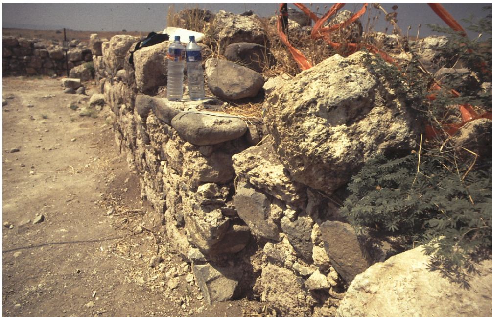
Figure 3: Faulted wall of the Ottoman mosque. Picture taken in 1994, before the excavation.
