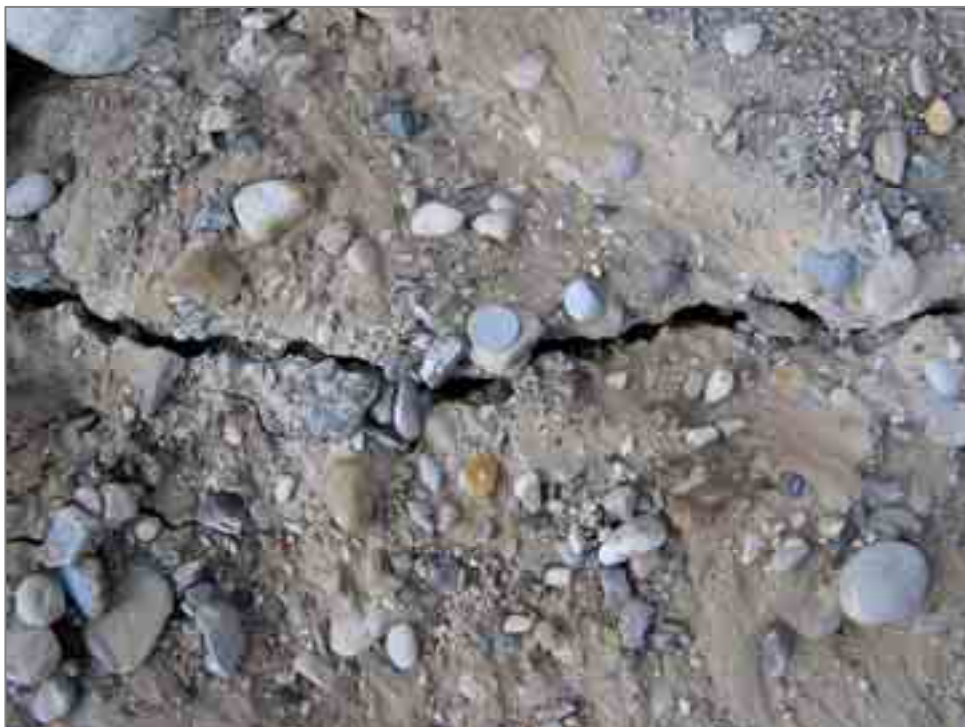
Photo 3. Open cracks with vertical offset, probably due to differential compaction, in the N. Darga gully near its outlet to the sea. The cracks are oriented oblique to the shoreline.
