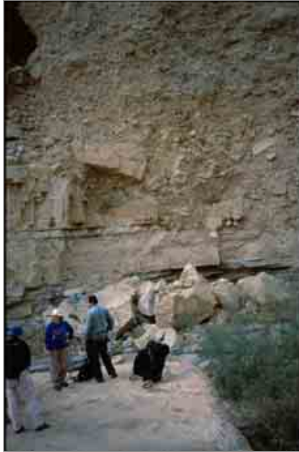
Photo 9. Collapse of fractured hard carbonate rocks of the Judea Group and talus, N. Arugot. Photo was taken in the afternoon, after the earthquake.
