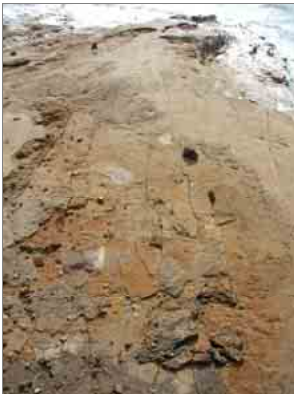
Photo 4a. Re-opened cracks along the Qalya coast. Pattern of cracks is oblique to the shoreline. Photo was taken the day after the earthquake.
