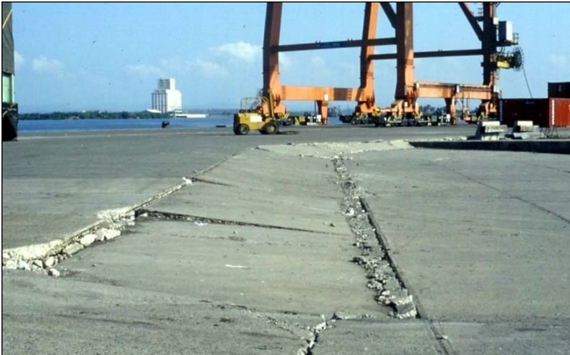
Figure r – September 19, 1985 Michoacan (Mexico) earthquake ( M_s 8.0): backfill compaction in the harbour facilities of Lazaro Cardenas. Photo E. Vittori.
