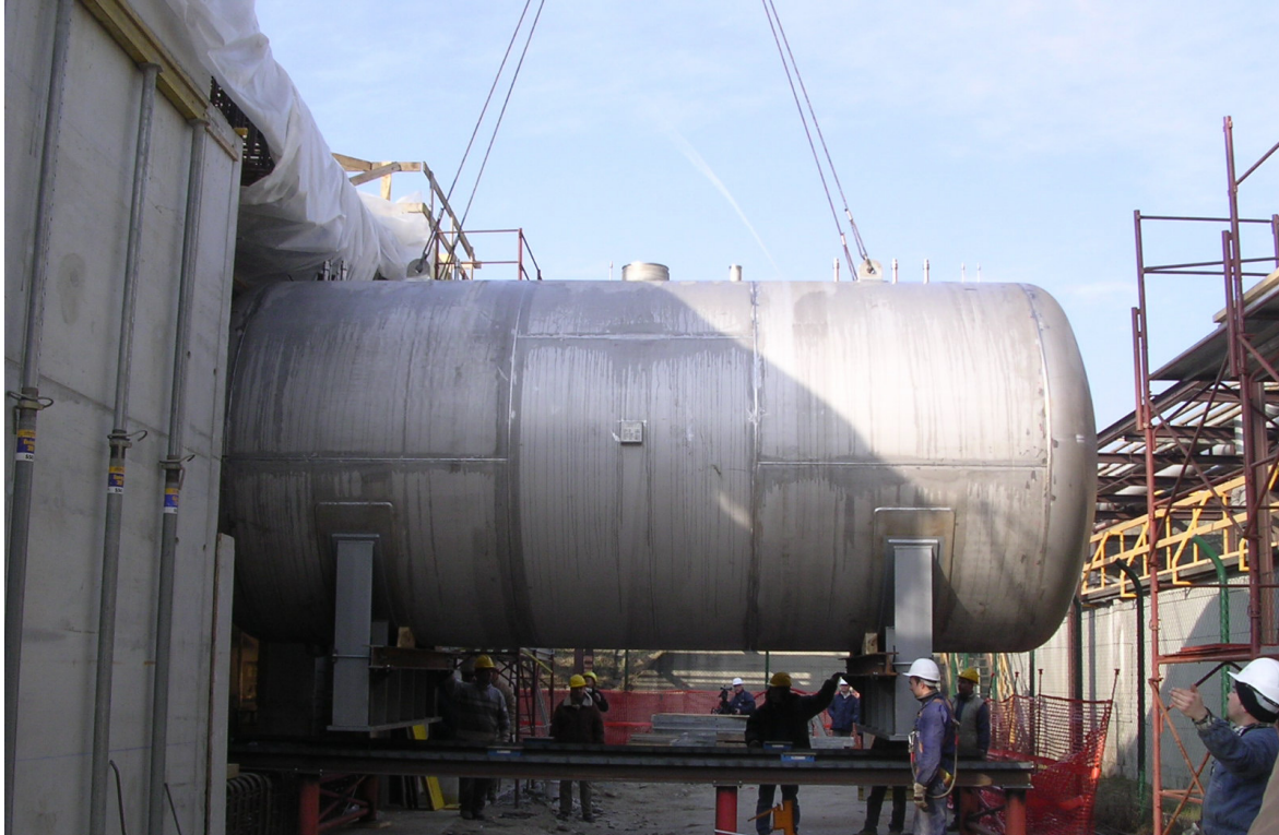
Figure 5: EUREX – One of the tanks of the new storage facility for High level Liquid Waste under construction
