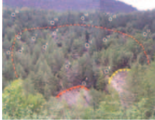
Figure. 18 - General view of Gardiola landslide; white circles identifies the target reflectors’ position.
