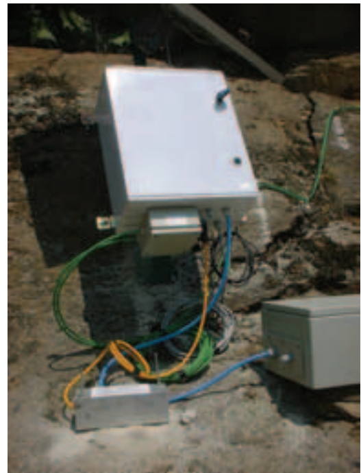
Figure 17 - Particular of micro-seismic data logger.
