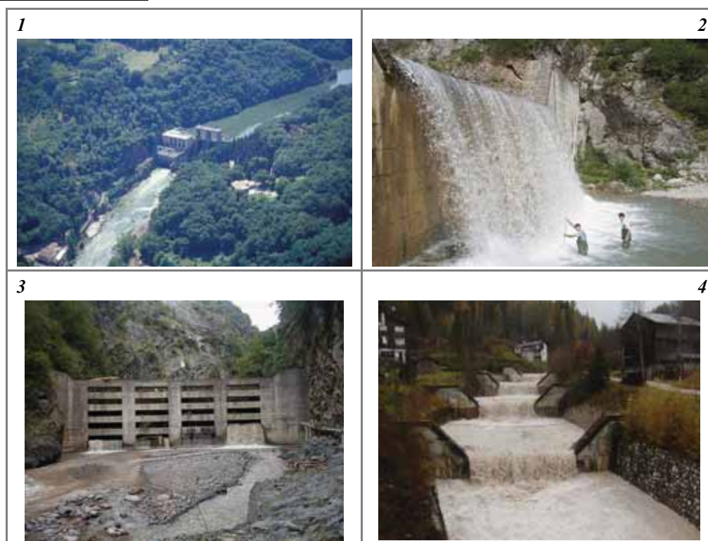
Figure 55 – Transversal structures of alteration of sediment discharges in mountain areas. (1) Dam; (2) retention check dam; (3) open check dam; (4) sequence of stepped consolidation check dams.
