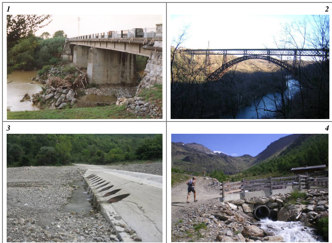
Figure 63 – Crossing structures. (1) Bridge with interference on fluvial dynamics; (2) crossing structure unrelated to the fluvial corridor; (3) ford with culverts; (4) culvert.
