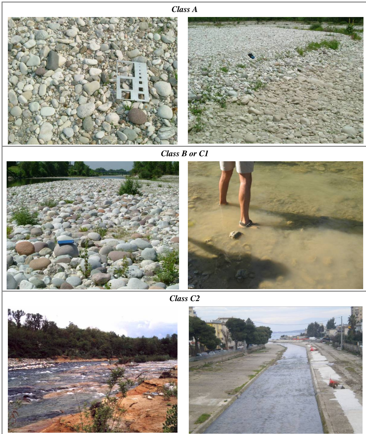
Figure 44 – Alterations of substrate in semi- and unconfined channels. Class A : natural sediment heterogeneity in an unconfined channel. Class B or C1 : presence of armouring (photo on left) or clogging (photo on right) (assignment to Class B or C1 will depend on the extension of armouring and/or clogging along the site). Class C2 : bedrock outcroppings due to bed incision (photo on left) or completely altered substrate because of bed revetment (photo on right).
