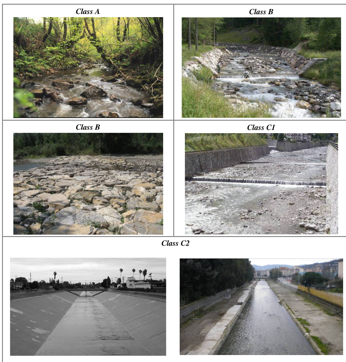
Figure 73 – Other grade control structures and revetments. Class A : total absence of other grade control structures or revetments. Class B : presence of sills (first row on right) or mass ramps (second row on left) with low density. Class C1 : various sills and partial bed revetment. Class C2 : total bed revetment with impermeable systems. If such revetments occur along most of the reach (> 80%), an additional score of 12 is assigned.
