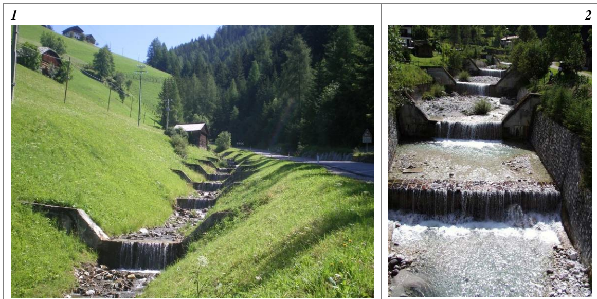
Figure 62 – Cases with very high density of transversal structures ( > 1 every 100 m in mountain areas): an additional score of 12 is applied.
