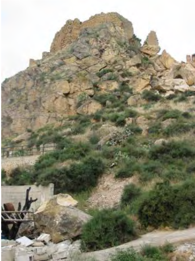
Figure 4.2.1b: View of south lateral of the easternmost point of the castle cliff and of the block that damaged a small wall of a house. The down-the-hill road pavement showed moderate damage at this point. It can be observed on the left the ending of the retaining wire mesh that stabilises the south face of the castle cliff.
