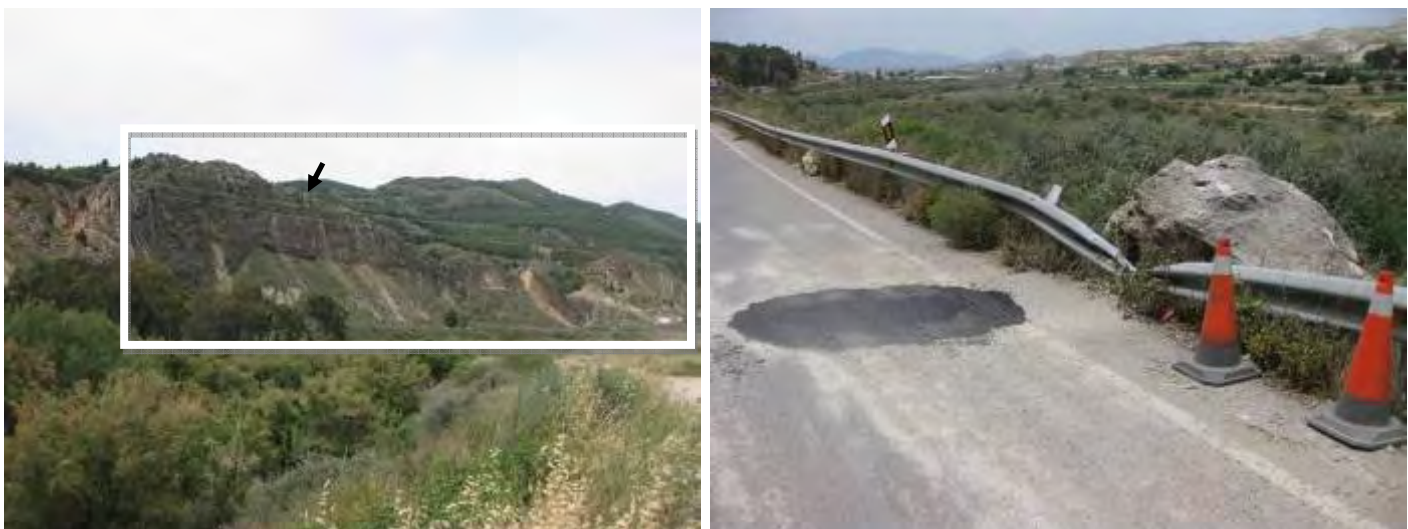
Figure 4.4.1b: Continuation of the Pantano de Puentes road towards the west. Along this road many instabilities were identified, although of a small size in general. Particularly remarkable are the rock blocks fallen from the ridge controlled by Las Viñas Fault (marked with an arrow). Picture on right shows a close-up of the damage produced by one of this rock blocks.
