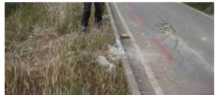
Figura 4.2.1d: Moderate damage on the down-the-hill road caused by the rebound of the block detached from the easternmost point of the cliff (figure 1.b).
