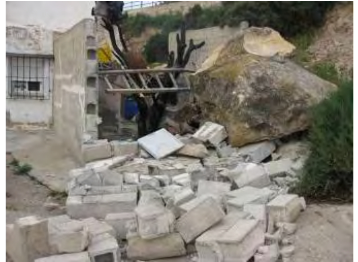
Figure 4.2.1c: Result of the impact on a wall made of concrete blocks enclosing the patio of a house from a rock detached form the easternmost pint of the cliff.
