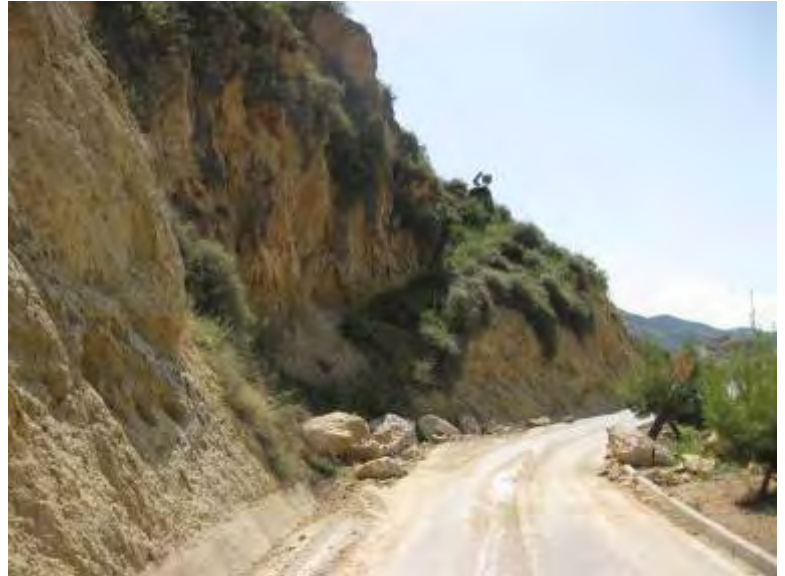
Figure 4.2.3: Rock-falls and debris on the up-the-hill road to the castle.
