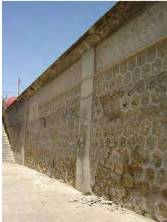
Figure 3.1. Masonry wall along Guadalentín river bank passing through Lorca, used as a marker.
