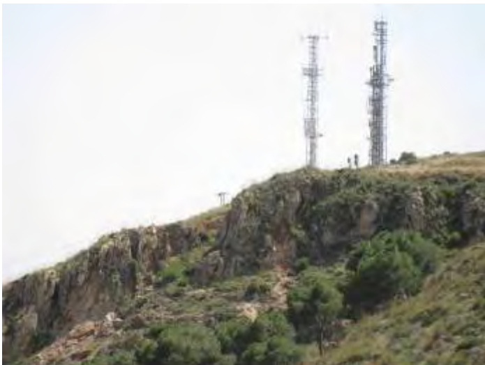
Figure 4.5: Communications towers founded on a hill situated in front of the westernmost end of Lorca's castle cliff. Two recent instabilities are shown, which are attributed to the 11 May earthquakes.
