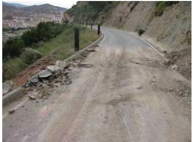
Figure 4.2.4b: Damage on the pavement of the up-the-hill road to the castle due to the fall and rebound of the block shown in figure 1.4a.
