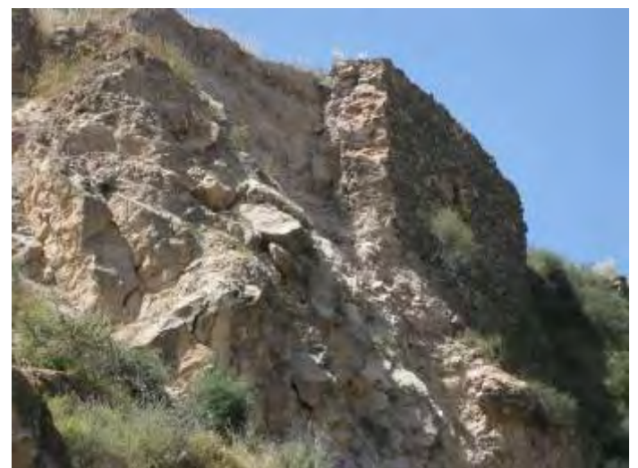
Figure 4.2.1f: Close up of the fall of part of an old retaining wall. It can be observed that the intrados filling remains meta-stable. This type of instability also appears on the south face of Lorca's castle cliff (see figure 2.1).
