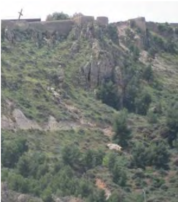
Figure 4.2.4a: Rock-fall of metric size that damaged badly the road (see figure 1.4b).
