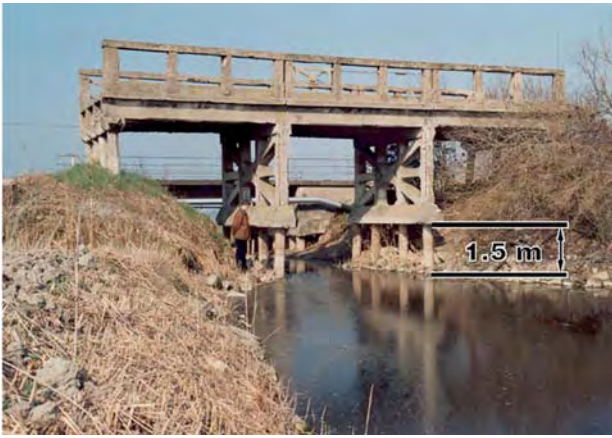
Fig. 94 – A bridge built in 1920s near the southern edge of lagoon at Chioggia, that is now protruding about 1.5 m due to oxidation of surrounding peat soils (from TOSI et alii, 2000).
