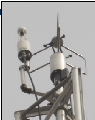
Gas analyser & Sonic anemometer
