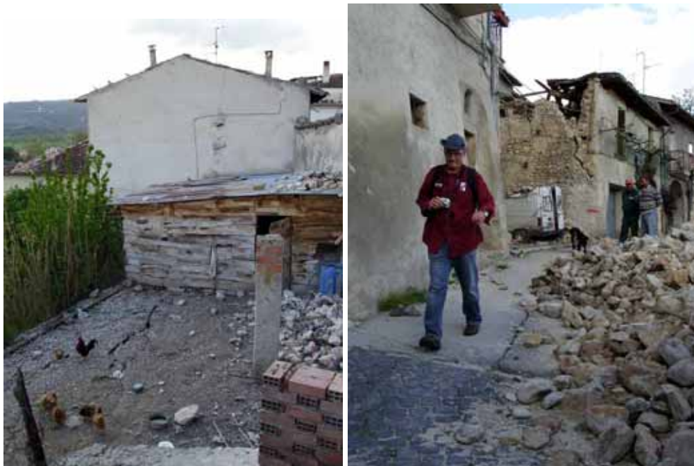
Fig. 18. Fractures in buildings and paved road at Paganica, Via delle Volpi.
