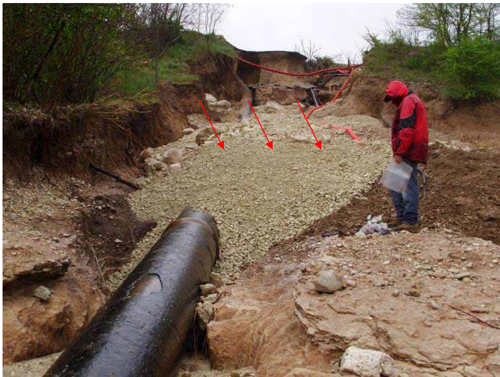
Fig. 11 - The site where the aqueduct was broken. The location of ground ruptures (before being covered) is pointed out by red arrows
