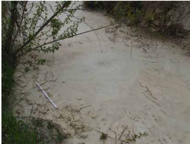
Fig. 40 – Liquefaction in artificial material in the industrial area of Bazzano
