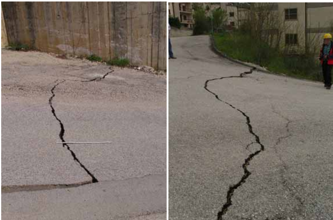
Fig. 13. Fractures in paved roads in Paganica some tens of meters east of the broken aqueduct
