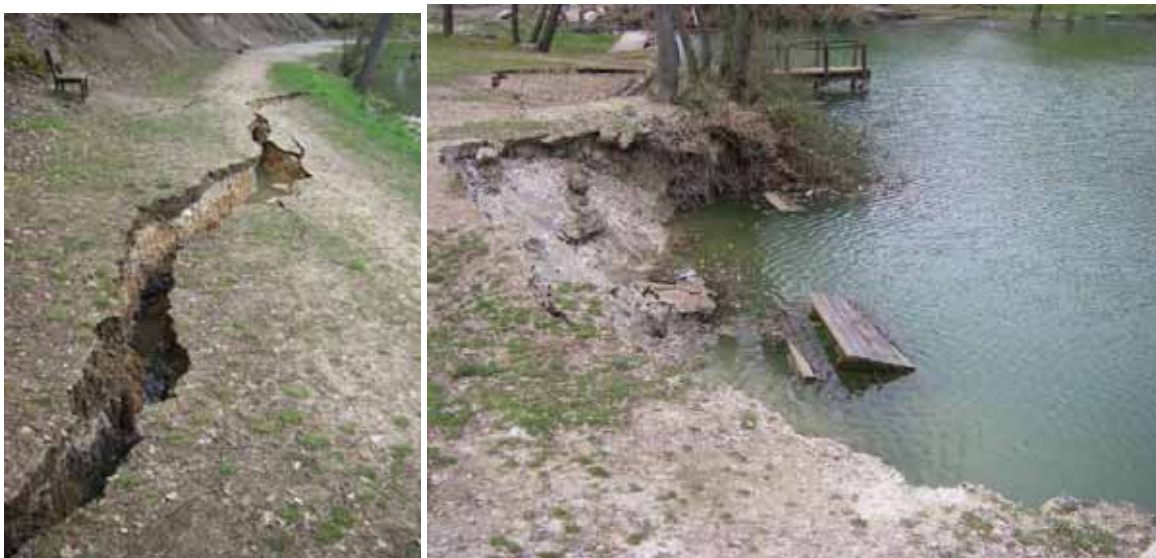
Fig. 36 – Ground failures along the shorelines of Lake Sinizzo banks
