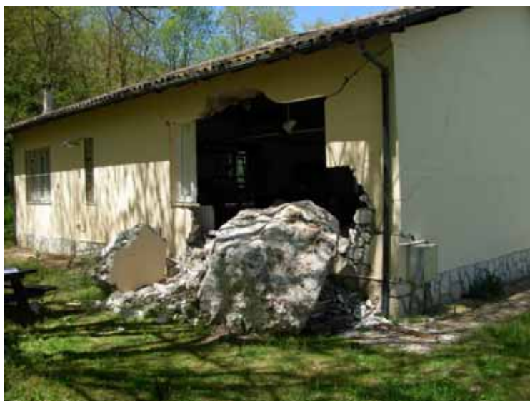
Fig. 32 – A huge block damaged the cafe near the entrance of the Stiffe Cave
