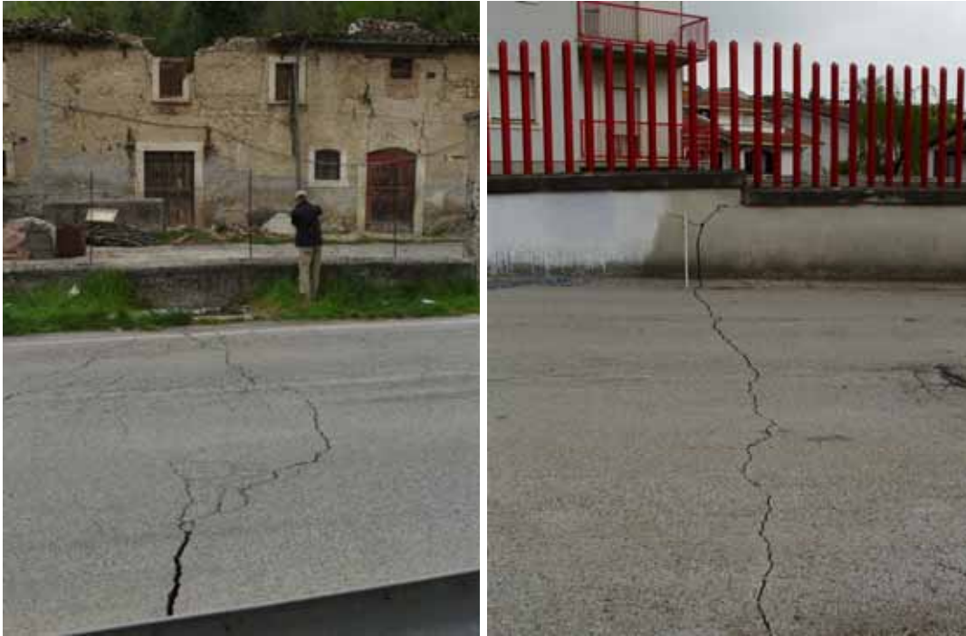
Fig. 15. The ruptures were clearly visible also on the road from Paganica to Camarda.
