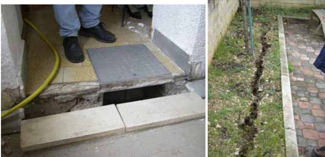
Fig. 14. Two ruptures affecting a modern building and a house-yard in Paganica
