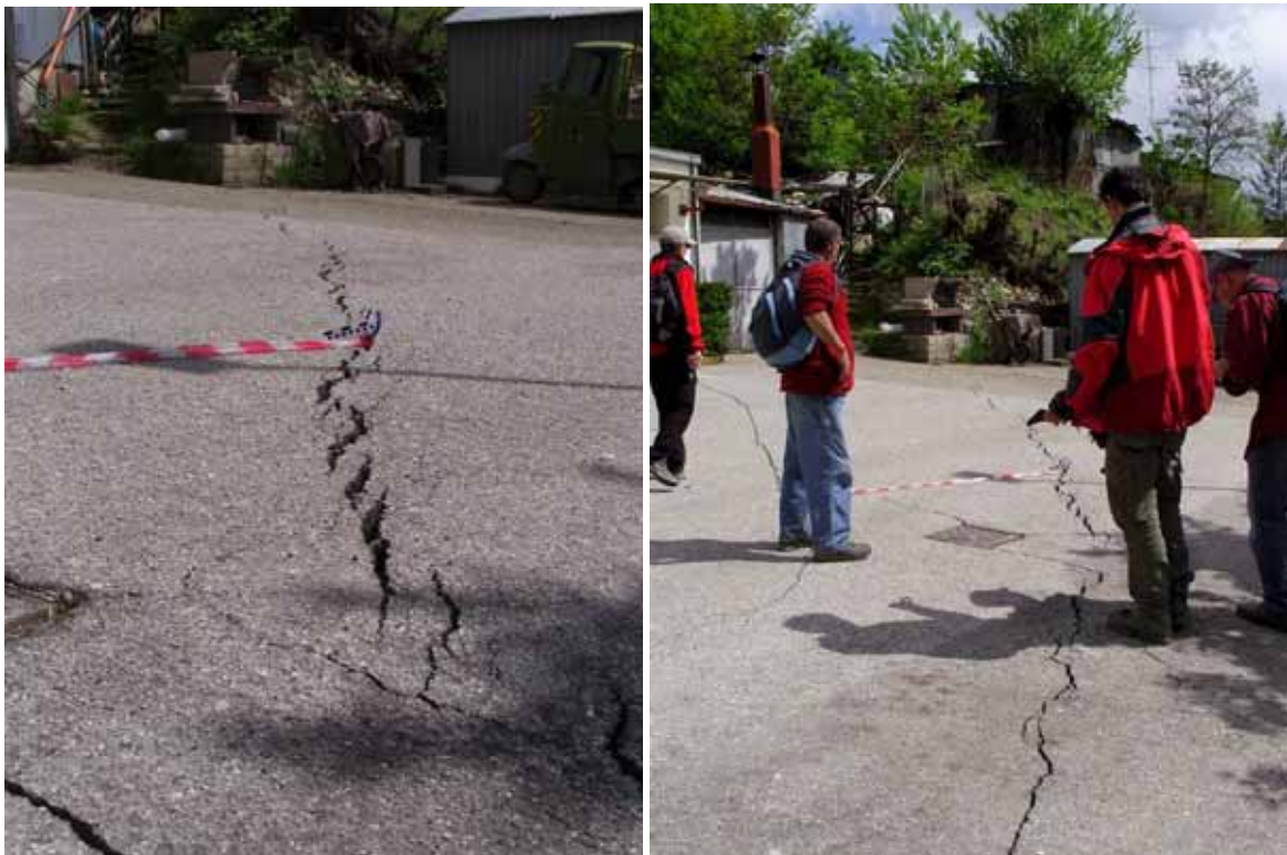
Fig. 16. Fractures in paved roads at Paganica, Via del Caldarello
