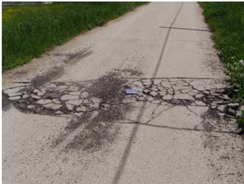
Fig. 39 – Fossa: fractures in paved road near a bridge on the Aterno River.
