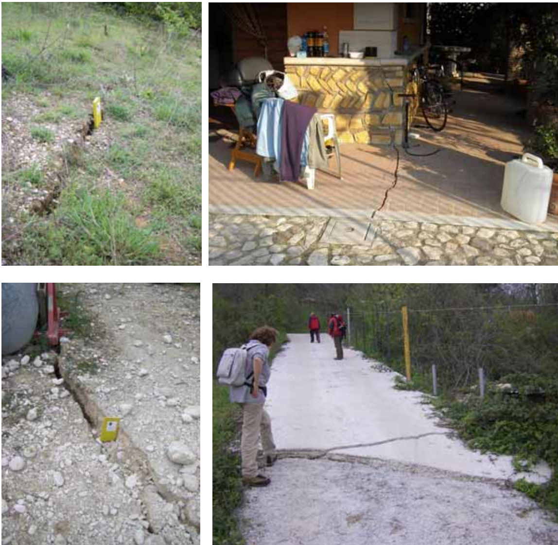
Fig. 15. The ruptures affected the ground, some buildings and concrete roads continuously for several hundreds of meters with offsets up to 7-8 cm.
