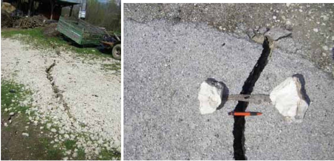
Fig. 38 – Onna: fractures in artificial material and in paved road near a bridge on the Aterno River.
