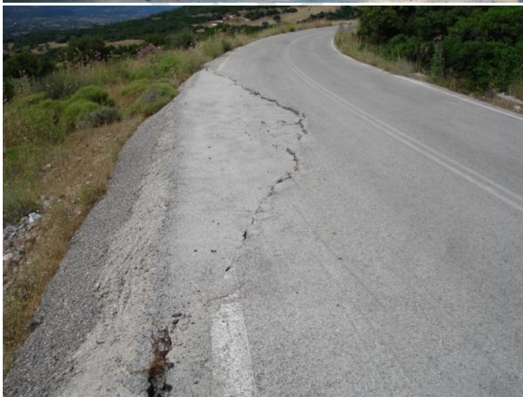
Figure 13. Road failure due to slope movement between Santoneri and Portes.
