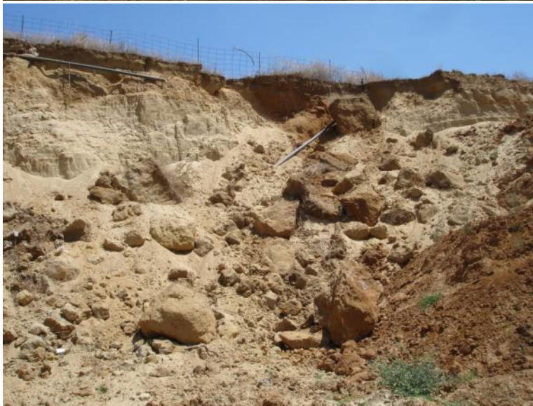
Figure 15. This slope failure exposed and damaged the irrigation pipe.
