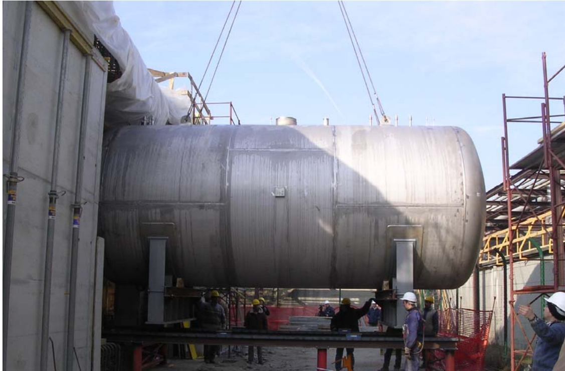
Figure 5: EUREX – One of the tanks of the new storage facility for High level Liquid Waste during the construction
