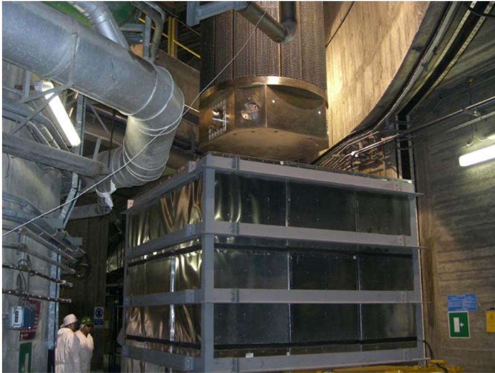
Figure 7: Caorso NPP – A phase of spent fuel transport casks handling inside the reactor containment with a special shock absorber structure
