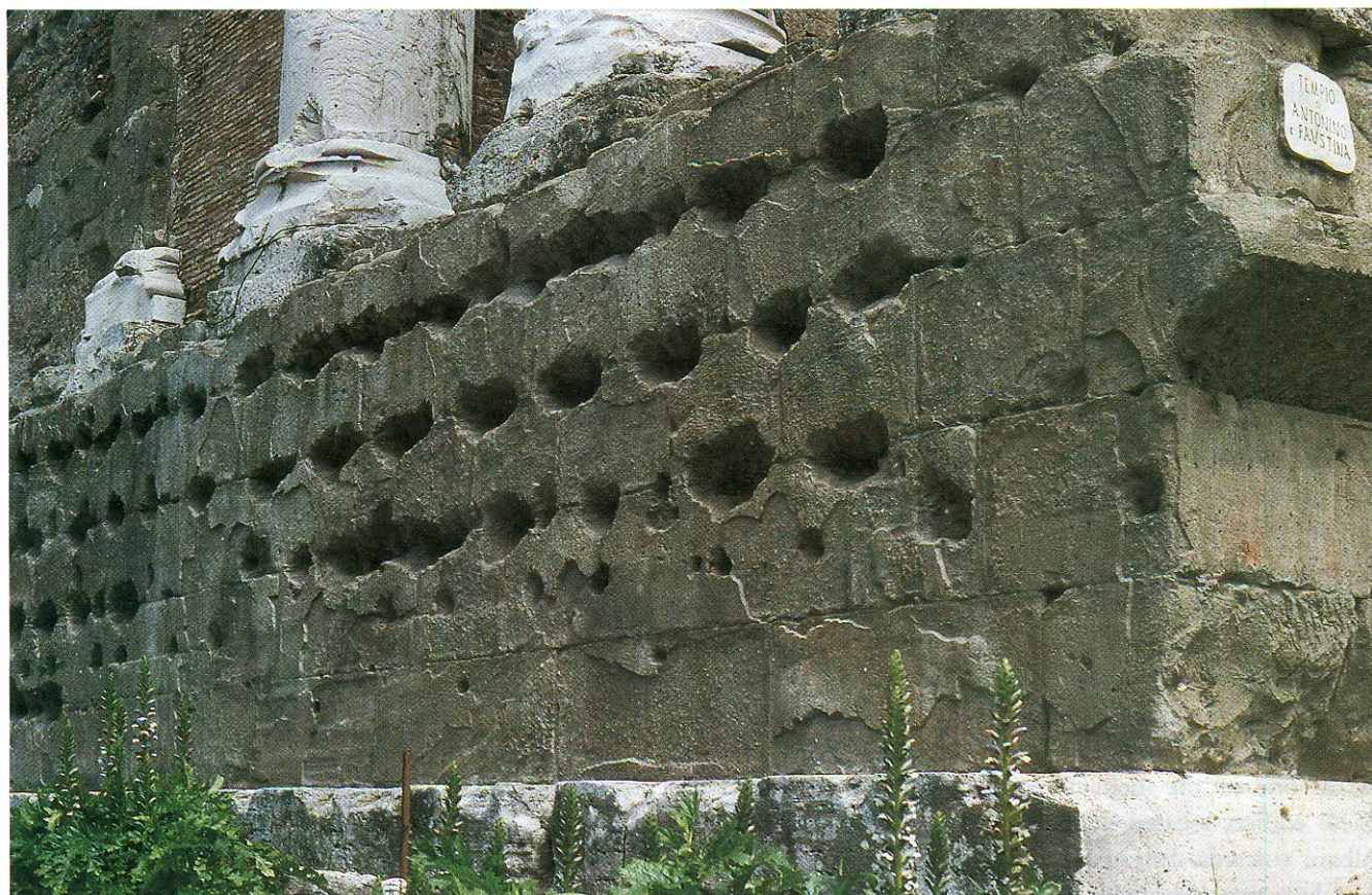
Fig. 6. – Foro di Cesare; the Antonino and Faustina temple whose basal structures are made with lapis Albanus.
