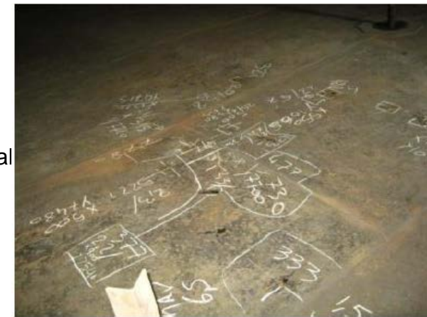
Photograph 7: Tank bottom is subject ail to internal as well external corrosion.
