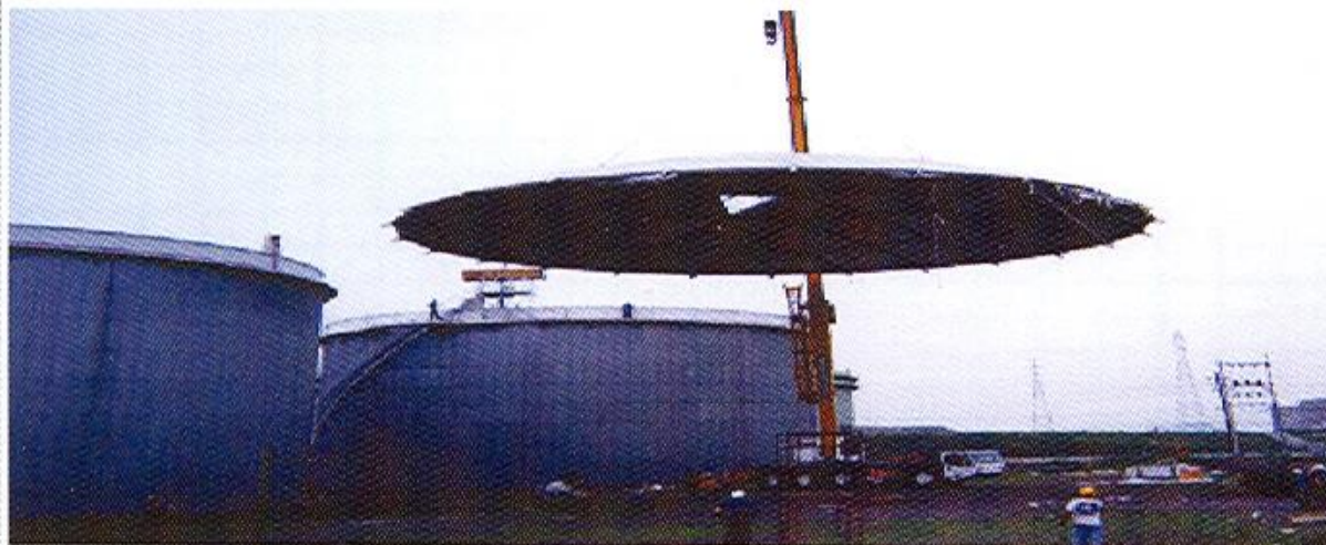
Erection Works of Petroleum Storage Tank Dia. 35m Al. Dome Roof for Local Oil Refinery
