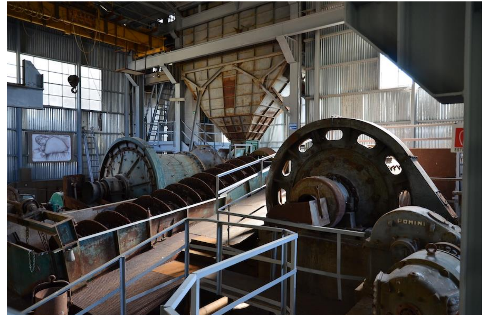
Interior of the Sos Enattos processing plant (laveria), equipped with crushers, mills, spiral separators, and a flotation system.
